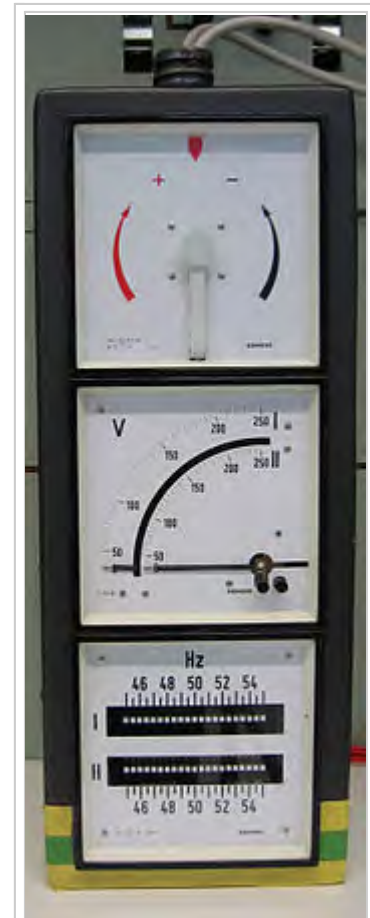
From top to bottom: synchroscope, voltmeter, frequency meter. When the two systems are synchronized, the pointer on the synchroscope is stationary and points straight up.
