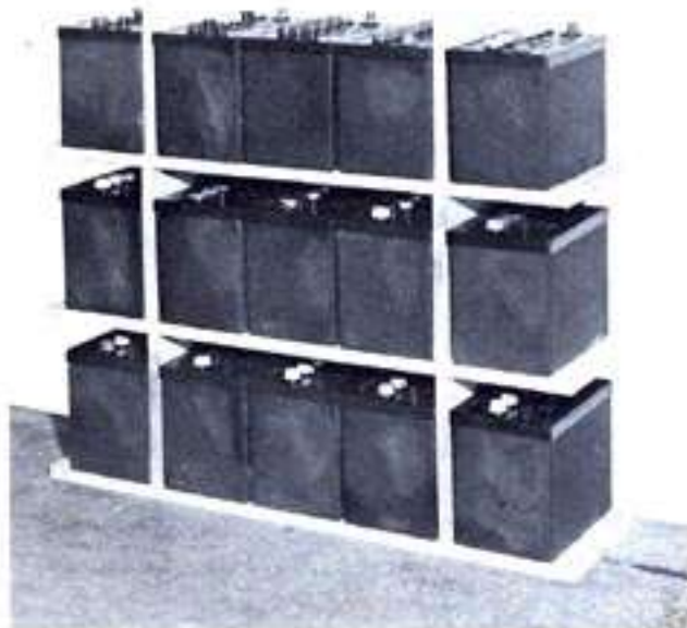
Fig. 24—Battery Storage Rack.
