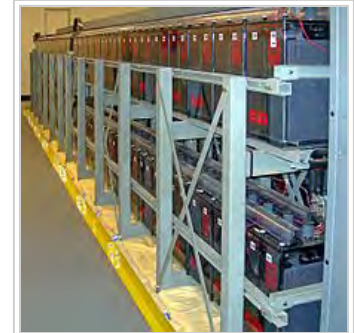
A battery bank used for an uninterruptible power supply in a data center
