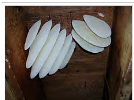
New wax combs between basement joists
