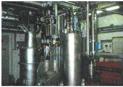
Wood gasifier for co-gen set
