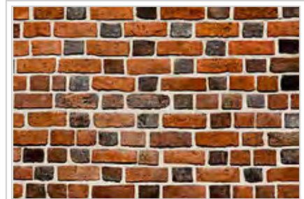
A wall constructed in glazed-headed Flemish bond with bricks of various shades and lengths
