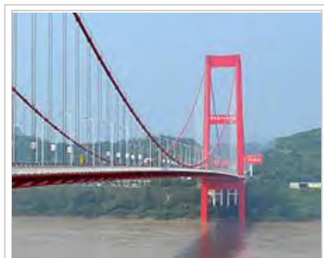
The Yichang Bridge, a plate deck suspension bridge, over the Yangtze River in China
