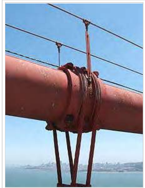
Suspender cables and suspender cable band on the Golden Gate Bridge in San Francisco. Main cable diameter is 36 inches (910 mm), and suspender cable diameter is 3.5 inches (89 mm).
