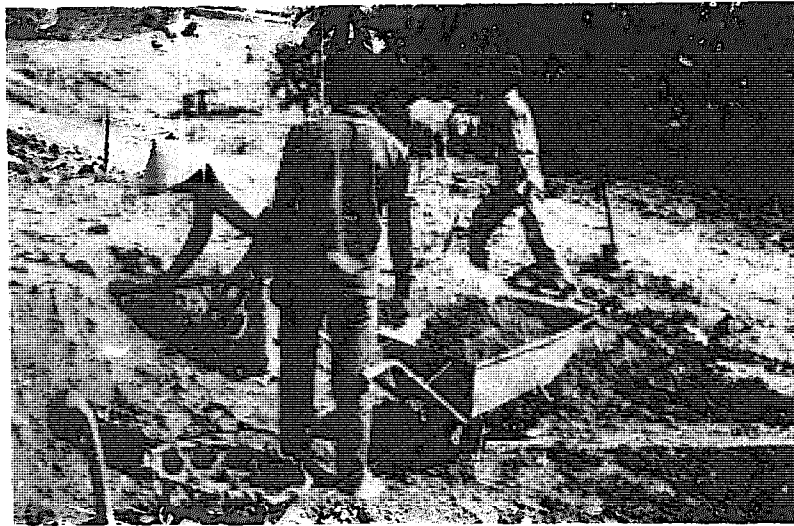
Figure 2. WESTERN-STYLE BARROW, LOCALLY AVAILABLE IN INDONESIA, USED IN CANAL CONSTRUCTION STUDIES (Weight 16kg Payload 75kg)
