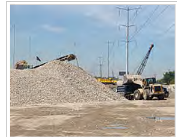
Recycled crushed concrete, to be reused as granular fill, is loaded into a semi-dump truck.
