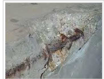
Concrete spalling caused by the corrosion of rebar
