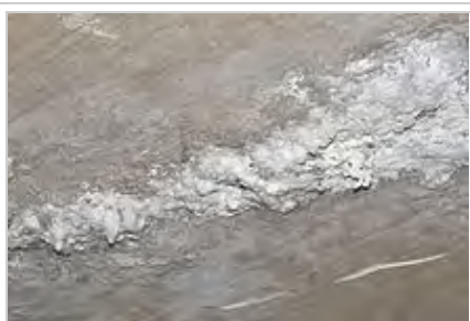
Example of secondary efflorescence in parking garage exposed to diluted road salt from vehicles entering the garage during winter.
