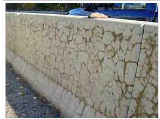
Typical crack pattern associated to the alkali-silica reaction affecting a concrete step barrier on a US motorway (photograph, courtesy of the Federal Highway Administration (US Department of Transportation).
