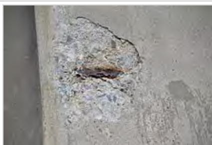
Example of flat piece of concrete having dislodged with corroded rebar underneath, Welland River bridge across Queen Elizabeth Way in Niagara Falls, Ontario.
