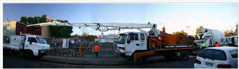
Because it is a fluid, concrete can be pumped to where it is needed. Here, a concrete transport truck is feeding concrete to a concrete pumper, which is pumping it to where a slab is being poured.
