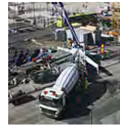
Fully deployed concrete pump, showing outriggers and boom in use while receiving concrete.
