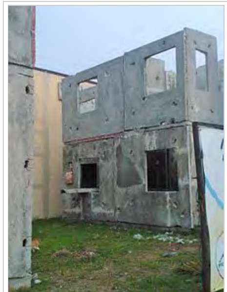
An example of low-quality precast concrete with exposed dowels, connectors and presence of cracks and malformations even during its installation.
