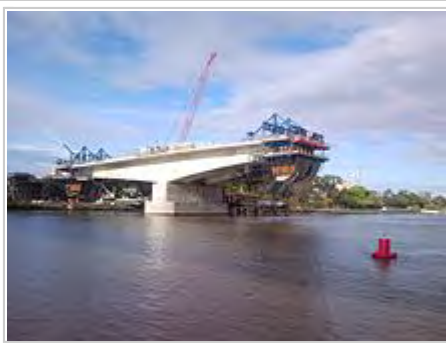
Balanced-cantilever bridge under construction. Each added segment is supported by post-tensioned tendons
