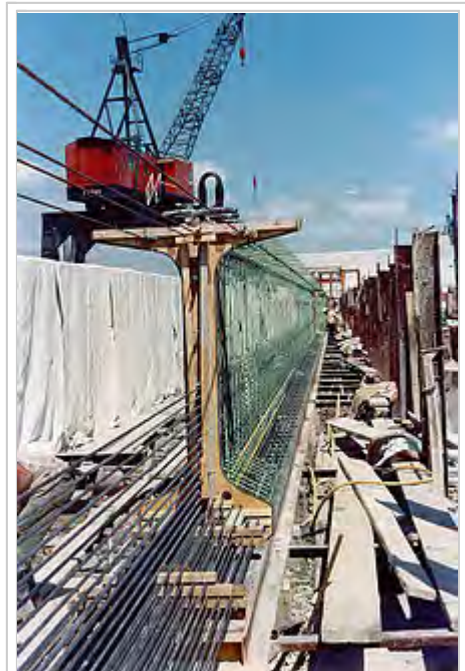
Pre-tensioned bridge girder in precasting bed. Note single-strand tendons exiting through formwork
