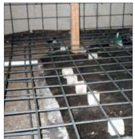
Figure 3. Concrete “dobies” are used to hold rebar off the ground or away from forms, ensuring adequate concrete coverage and preventing rust.
