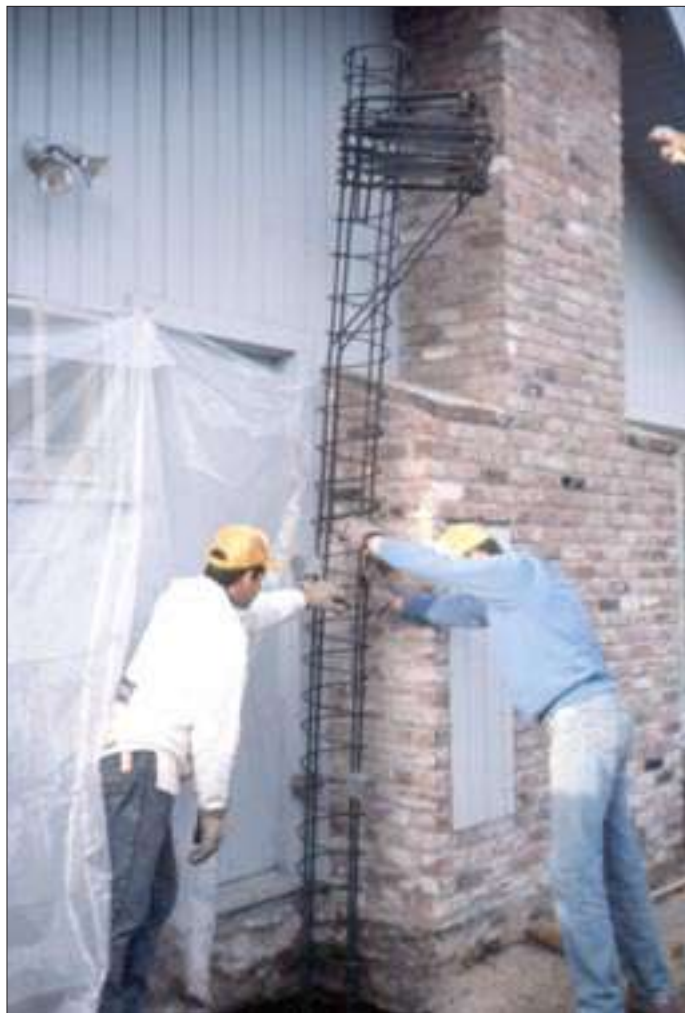
Figure 1. For deep concrete piers, the author uses steel cages made from #3 rebar spirals with #5 rebar in the middle. The cage shown here will help support the brick chimney in a foundation underpinning job.
