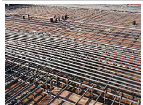
Rebar constructed to properly reinforce a beam element, awaiting concrete to be poured.
