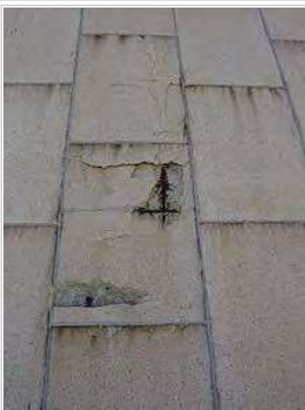
Detailed view of spalling probably caused by a too thin layer of concrete between the steel and the surface, accompanied by corrosion from external exposure
