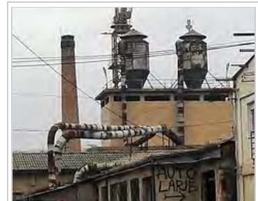
A dust collector in Pristina, Kosovo
