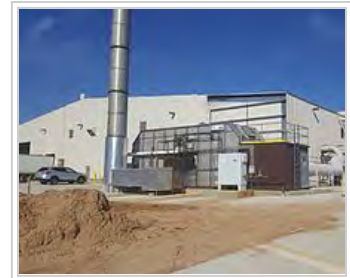
Air pollution control system, known as a Thermal oxidizer, decomposes hazard gases from industrial air streams at a factory in the United States of America.
