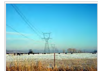
High voltage transmission lines deliver power from electric generation plants over long distances using alternating current. These lines are located in eastern Utah.
