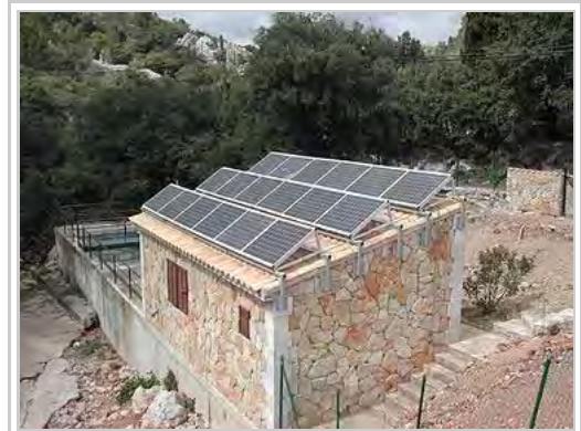
A sewage treatment plant that uses solar energy, located at Santuari de Lluc monastery, Majorca.
