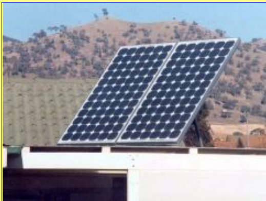
The solar panels on my roof. There are 2 more to come, for a total of 560 Watts.
