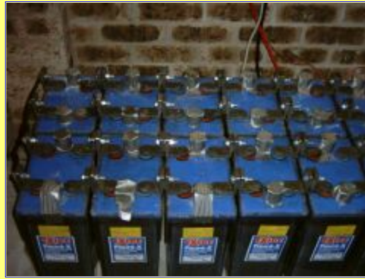
Half of the battery bank.
