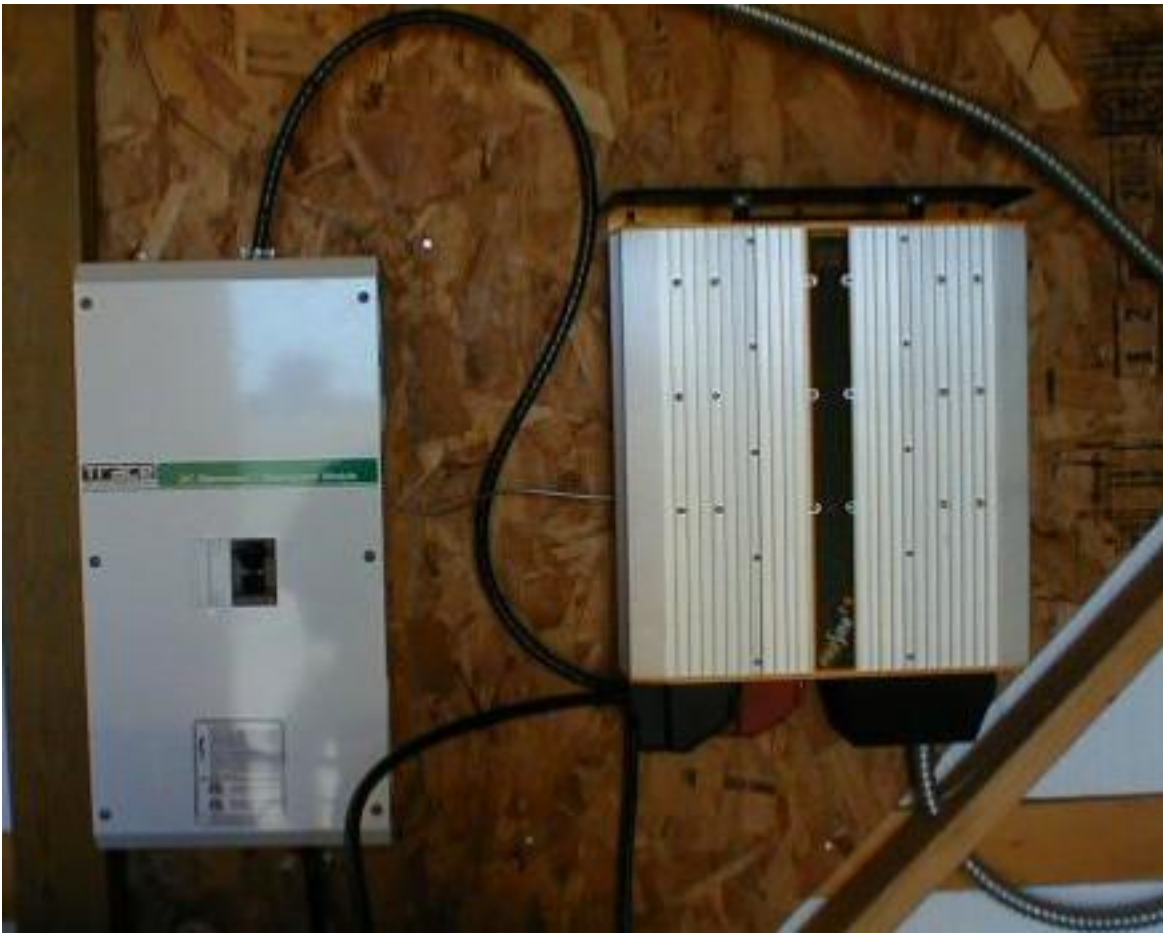
The Main disconnect box - 175 amps at 24 volts DC, and the 2.5Kw 24vdc/120vac inverter. This begins the 120 volt AC side of the system.
