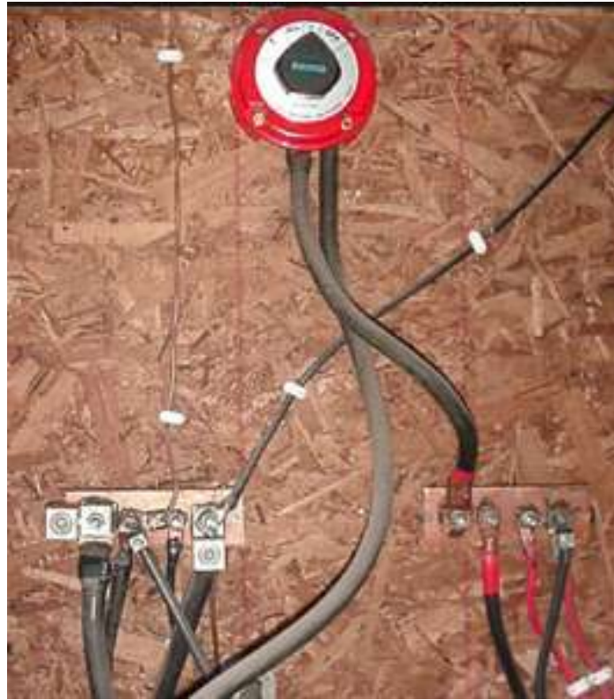
My buss bars and main power switch
