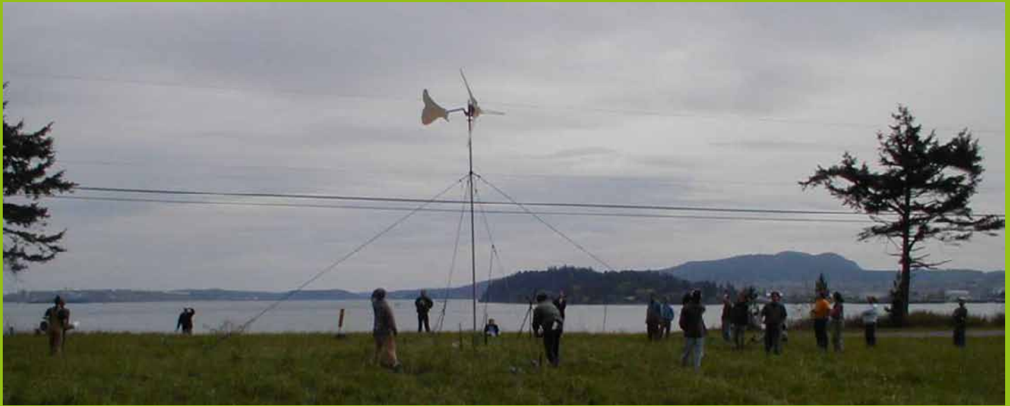
This is the bigger of the two machines we finished during the course. Rotor diameter is 8 feet (2.4 metres).
