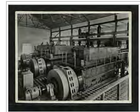
Three English Electric 7SRL diesel alternator sets being installed at the Saateni Power Station, Zanzibar 1955
