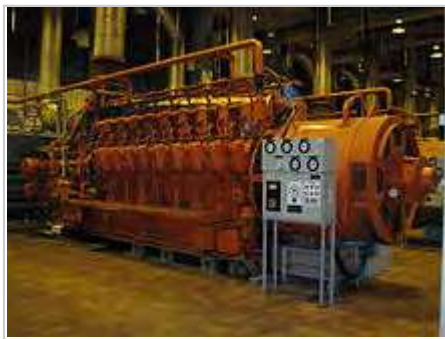
Big Diesel generator used for backup power
