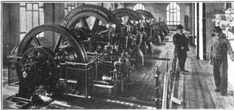
FIG. IV.—28. Six 300 H.P. Koerting four-cycle, single-acting, twin-engines at Julienhitte Electricity Generating Station.
