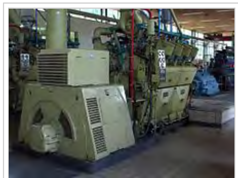
Brons two-stroke V8 Diesel engine driving a N.V. Heemaf generator.
