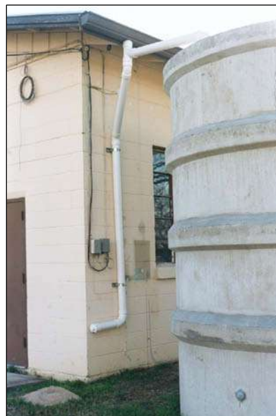
Stacked concrete ring 3,000-gallon tank at the Auld Center, Kerrville, showing first flush diverter and cistern.
