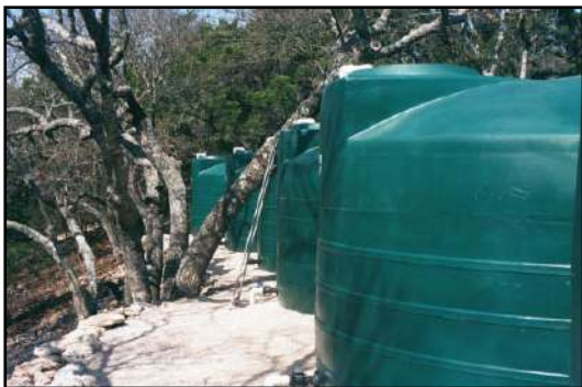
Figure 2-6. Low-profile 5,000-gallon polypropylene tanks
