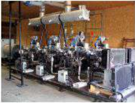
A better view of the six V8 engines driving the alternator seen at the rear, but not connected.
