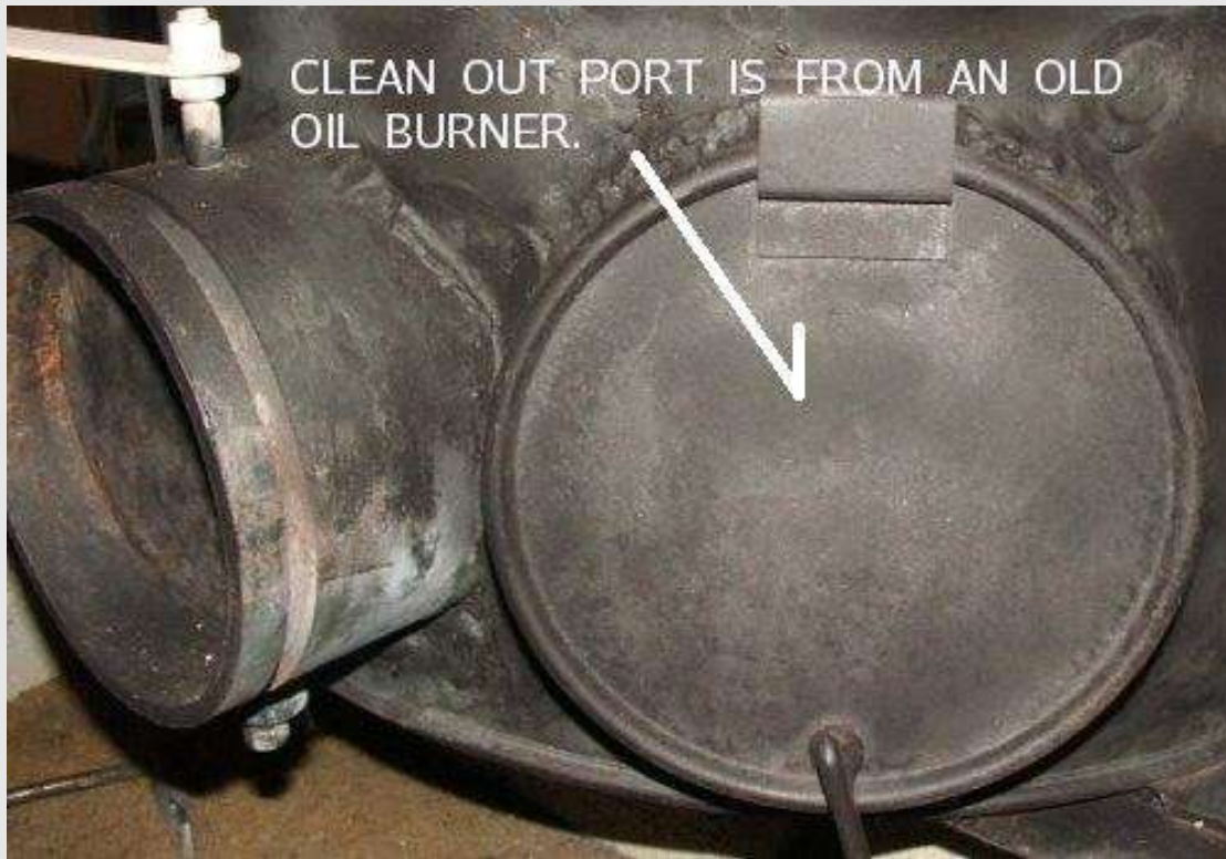
Main air and clean out ports.
