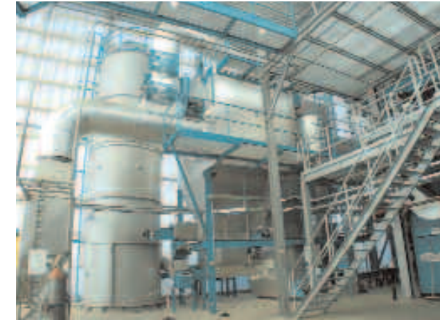
Figure 2: Flue gas cleaning.
