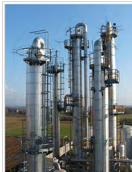
Typical industrial distillation towers
