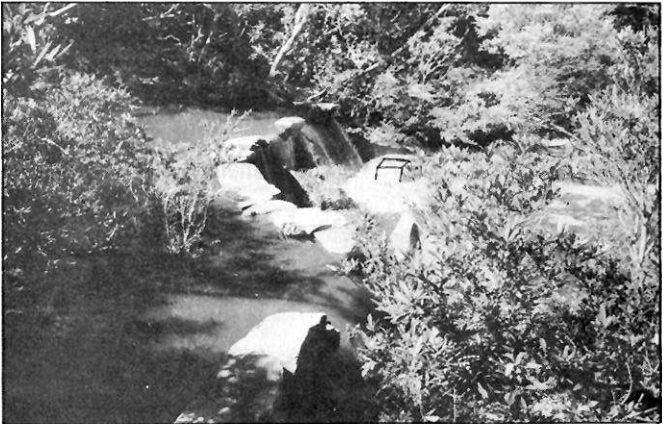
The pump and turbine were unaffected by this flood which totally submerged them both. The top half of the pump box is visible in the centre of the photo.
