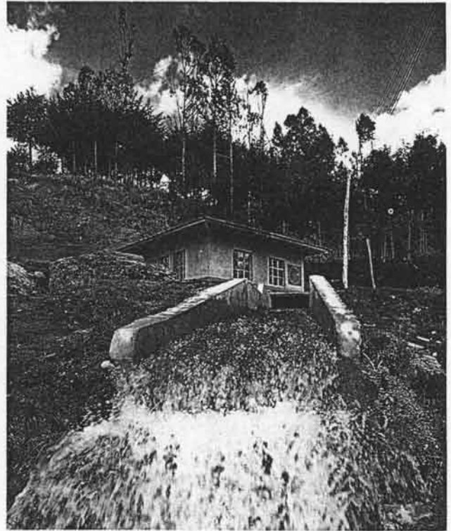
Powerhouse at Cajamarca (IT)
