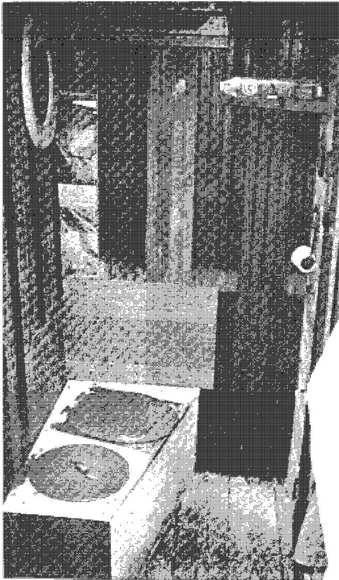
A PEAT TOILET WITH A RECESSED CONTAINER HOLDING PEAT MOSS FOR USE AS A COVER MATERIAL.
