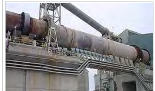
Hot end of medium-sized modern cement kiln, showing tyres, rollers and drive gear
