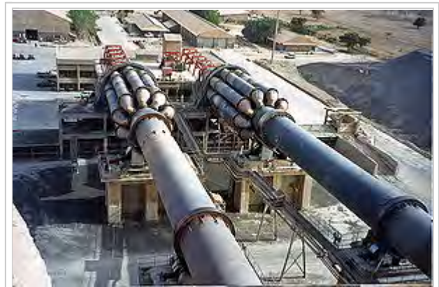
A pair of kilns with satellite coolers in Ashaka, Nigeria Sysy
