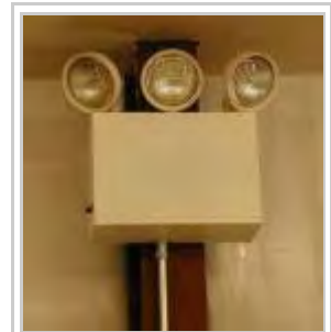
Three bulb emergency light in a residential building.
