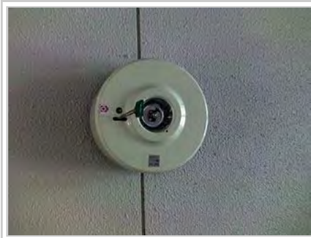
A small emergency light.
