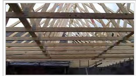
Joinery and roof trusses made from softwood
