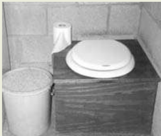
EMERGENCY SAWDUST TOILET IN BASEMENT OF NEW HOME WITH SEPTIC SYSTEM
