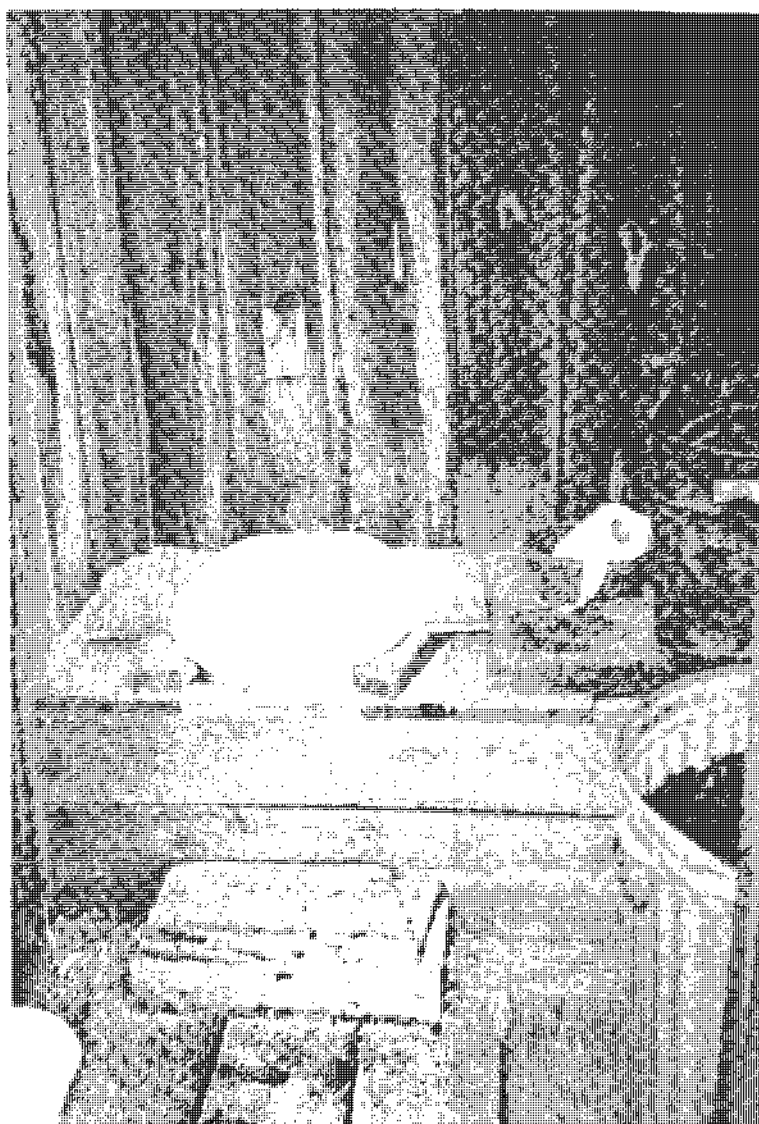
AN OUTDOOR SAWDUST TOILET BUILT OF RECYCLED MATERIALS. A REMOVABLE BUCKET LINGERS UNDER THE TOILET SEAT, WAITING TO BE FILLED, EMPTIED AND COMPOSTED.
