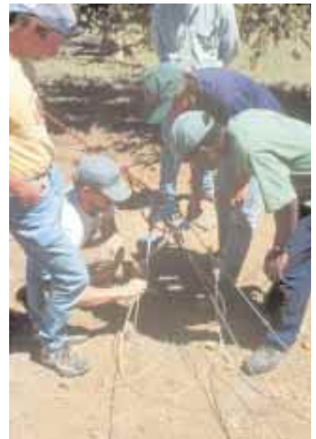
Untangling the maze of tower guy cables.
