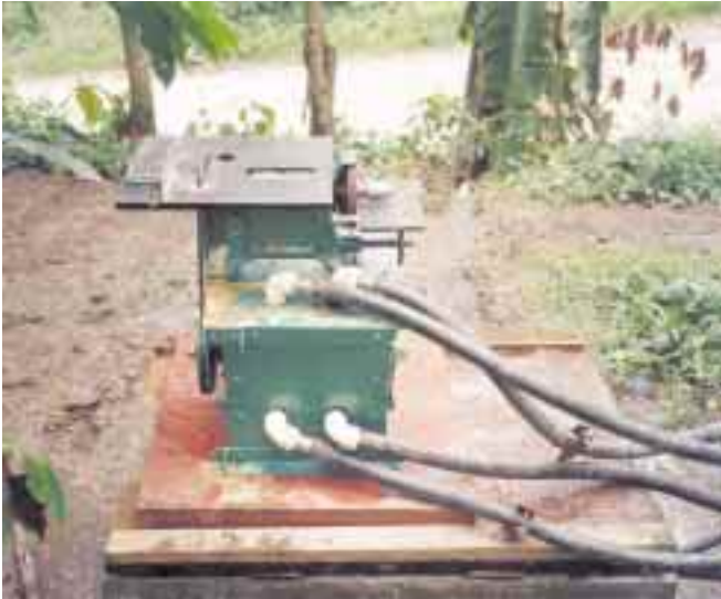
Plumbed to the power and ready to rip.
