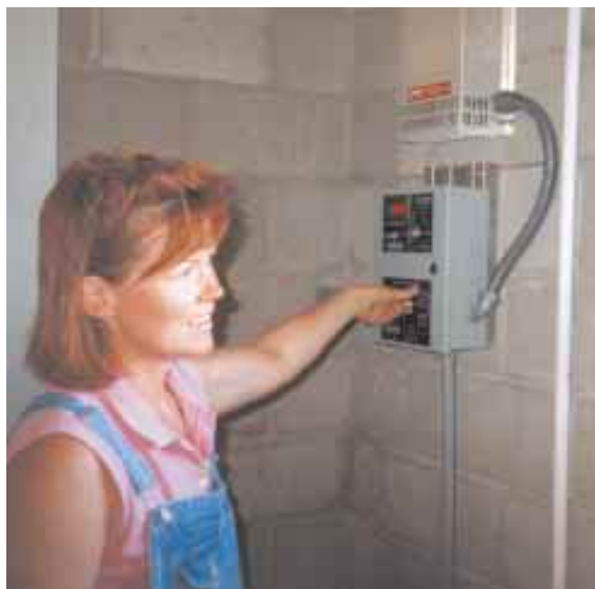
An enthusiastic Lou Ann throws the final switch, starting up the wind generator.
