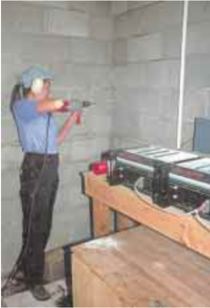
Drilling the battery room walls for tower wiring access. Note the original location of the inverters over the battery box.
