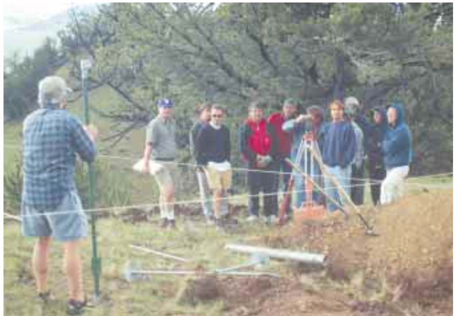
Johnny Weiss holds a makeshift surveyor’s staff while the crew checks anchor heights with a transit.
