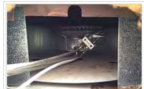
A thermocouple (the right most tube) inside the burner assembly of a water heater
