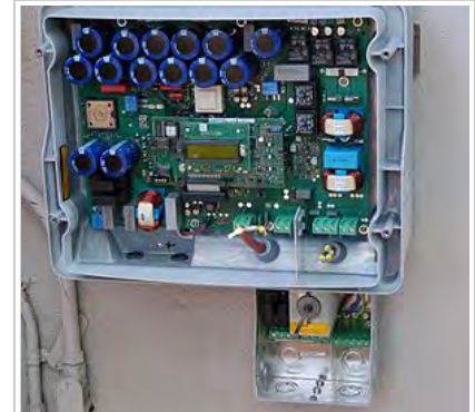
Internal view of a solar inverter. Note the many large capacitors (blue cylinders), used to store energy briefly and improve the output waveform.
