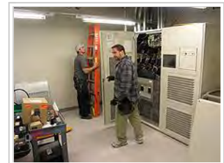
A large datacenter-scale UPS being installed by electricians
