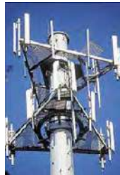
Sector antennas ( white bars ) on cell phone tower. Collinear arrays of dipoles, these radiate a flat, fan-shaped beam.
