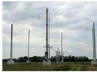
Quadrant antenna, similar to rhombic, at an Austrian shortwave broadcast station. Radiates horizontal beam at 5-9 MHz, 100 kW
