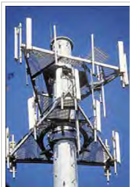
Cell phone base station antennas
