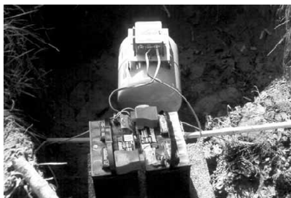
Figure 8. Pressure Tank and Batteries
