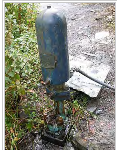
Figure 1: A hydraulic ram that drives a fountain at the Centre for Alternative Technology
