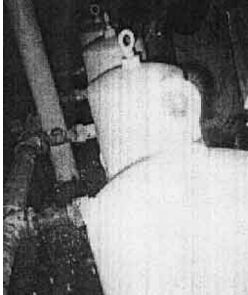
Fig.5 Renovated Adami-Tulu Hydraulic Ram Pumps
