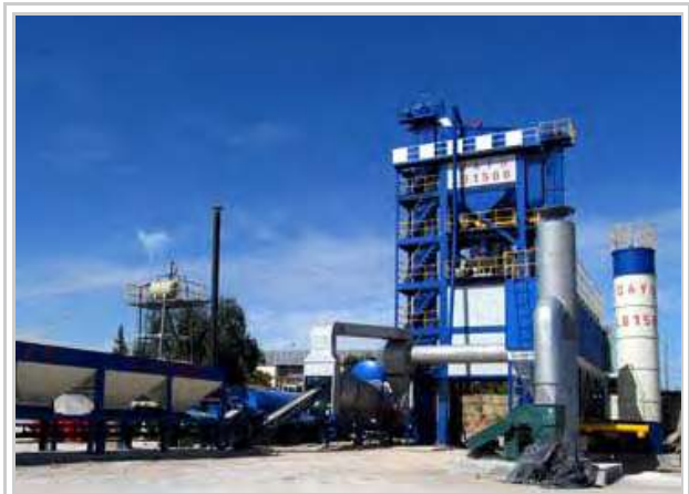
Asphalt batch mix plant
