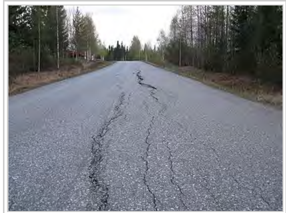
Asphalt damaged by frost heaves
