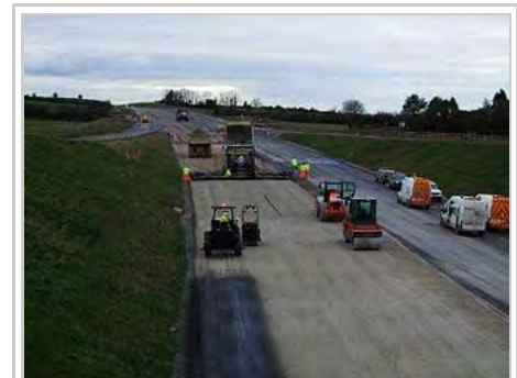
Sub-base layer composed of cement-based material being applied during construction of the M8 motorway in Ireland
