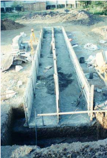
Figure 3-1 Construction of reedbeds, showing elevations of the floor. The outlet zone is in the foreground.
