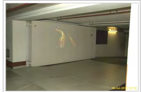
Large fire door, sealing a fallout and air raid shelter inside the basement parking garage of a hotel in Germany.
