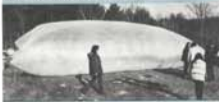
Sheet placed by Carroll team in single 20-by-100-ft. sheet of 3-mil polyethylene sheet makes and built dome.
