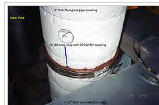
Fiberglass pipe insulation with ASJ (All Service Jacket) penetrating concrete slab opening about to be firestopped. Intumescent wrap strip is used to seal off where the fiberglass will be consumed by fire.
