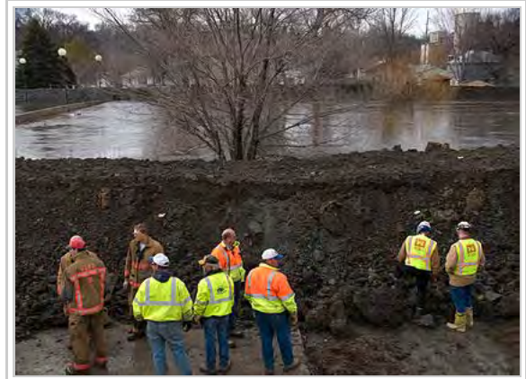
Slope instability issues for a temporary flood control levee in North Dakota, 2009
