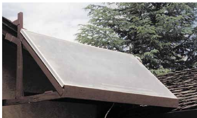
Figure 3: The solar thermal water panel.
