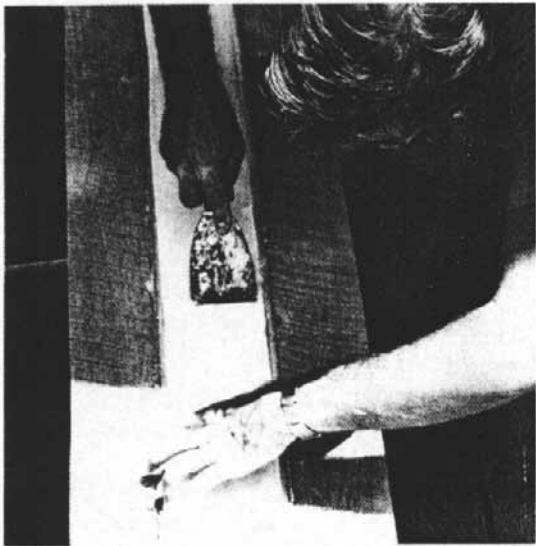
FIGURE 4.10—Smoothing out a new layer of silicone over the cloth, completely embedding the cloth (Skyheat Workshop photo).
